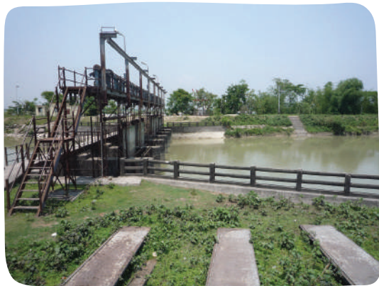
Fig. 8 - Sluice gates of Teesta Barrage in West Bengal.
